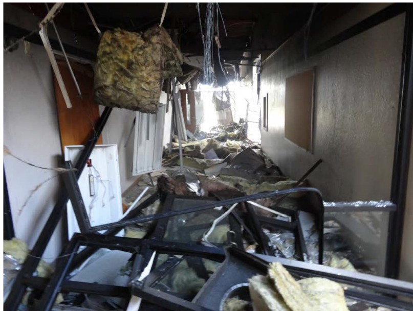
Damage at West Intermediate School
